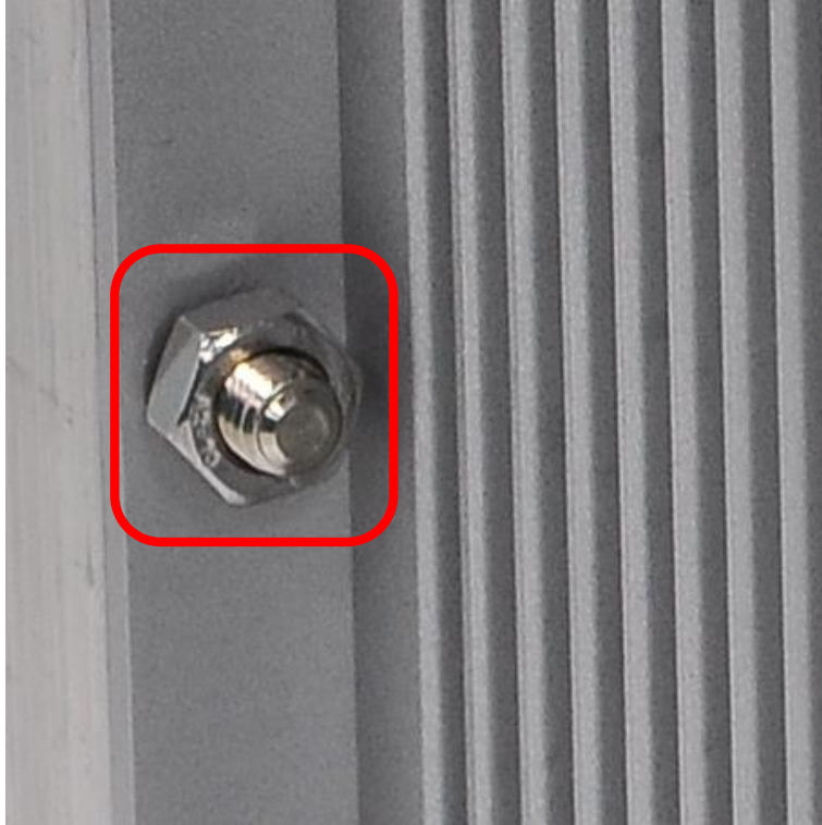
Ground screw of the switch
